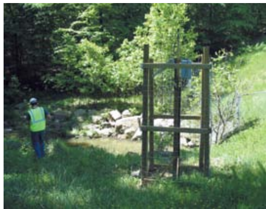
Water quality monitoring station installed by stream provides continuous data during construction project.
