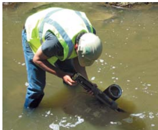
Contractor checks YSI water quality sonde at one of 63 monitoring locations set up around a large highway construction project.
