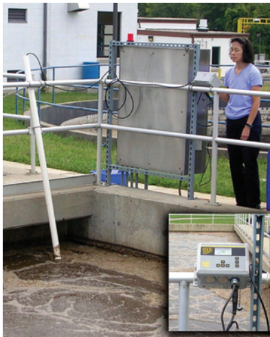
Dissolved oxygen measurement at an Ohio WWTP using a ROX optical sensor, multiparameter sonde, and process monitor.
