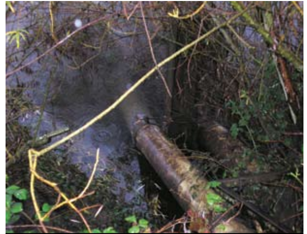
An intake pipe delivers water from the river to the nearby HydroSAM sampling system
