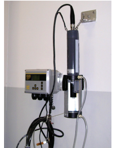
YSI 6920DW deployed at a water tower in Columbus, Ohio. The instrument, used in conjunction with a flow cell and a YSI 6500 Process Monitor, continuously monitors drinking water quality.
