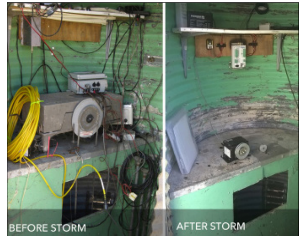
Inside of a Zone 7 Gage House Before and After Using Storm 3 and Storm Central
