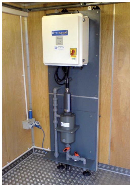
The compact HydroSAM provides long-term water quality monitoring for intake protection with less maintenance than larger systems. Shown here inside a protective shelter upstream of the water intake.
