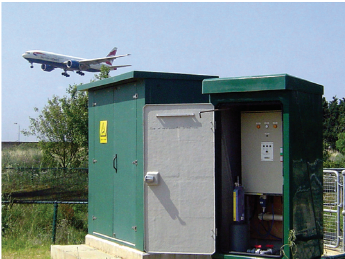
A WQMS pumping station with a YSI Sonde
